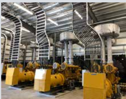
New Diesel Electrics
